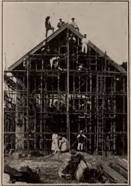
This is the way the Japanese carpenters build a house for our missionaries. Two lady teachers, Misses Hansen and Lindsey will live here.
